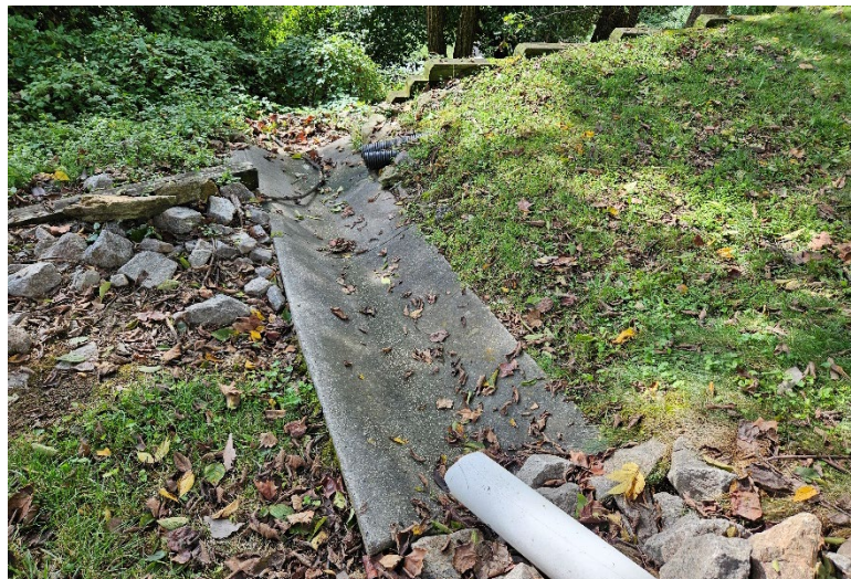
Photo 34: Roof Leader Discharge over the edge of Overlook Drive
