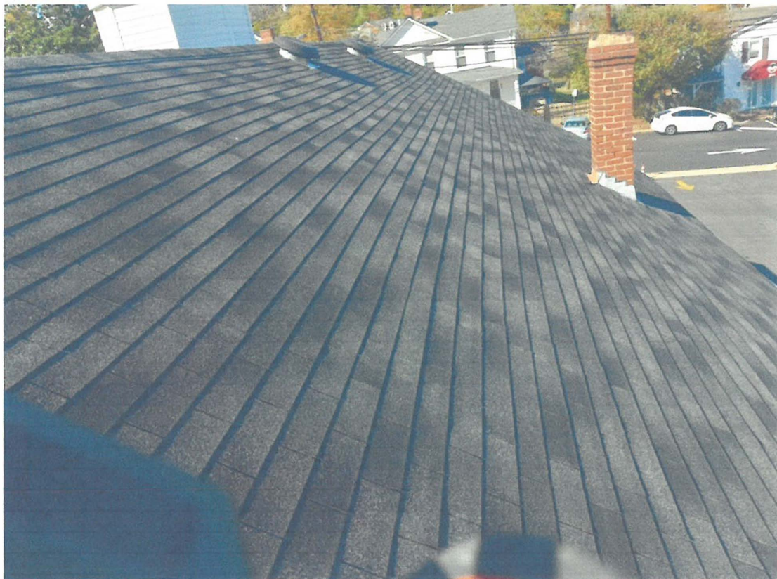
Most of shingles popping up due to soft/damage decking board underneath
